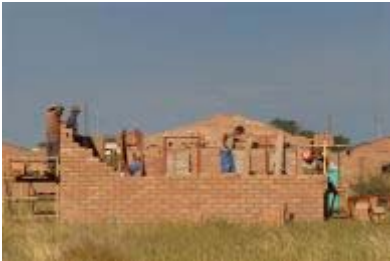
Upington, Northern Cape province: The Northern Cape Community Builders construct 100 low-cost houses. Photo: Graeme Williams, MediaClubSouthAfrica.com
