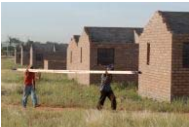
Upington, Northern Cape province: The Northern Cape Community Builders construct 100 low-cost houses. Photo: Graeme Williams, MediaClubSouthAfrica.com
