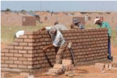
Upington, Northern Cape province: The Northern Cape Community Builders construct 100 low-cost houses. Photo: Graeme Williams, MediaClubSouthAfrica.com
