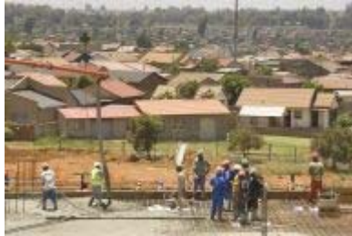
Johannesburg, Gauteng province: Construction on the new Natalspruit Hospital in Vosloorus, a large township in the south of Johannesburg.
