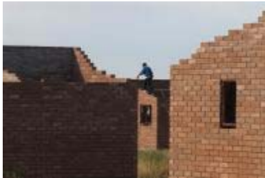
Upington, Northern Cape province: The Northern Cape Community Builders construct 100 low-cost houses. Photo: Graeme Williams, MediaClubSouthAfrica.com
