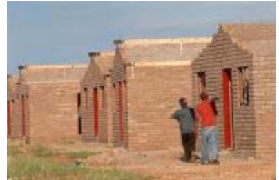
Upington, Northern Cape province: The Northern Cape Community Builders construct 100 low-cost houses. Photo: Graeme Williams, MediaClubSouthAfrica.com
