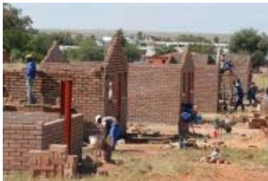
Upington, Northern Cape province: The Northern Cape Community Builders construct 100 low-cost houses. Photo: Graeme Williams, MediaClubSouthAfrica.com
