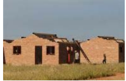
Upington, Northern Cape province: The Northern Cape Community Builders construct 100 low-cost houses. Photo: Graeme Williams, MediaClubSouthAfrica.com
