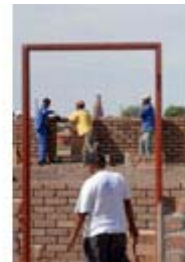
Upington, Northern Cape province: The Northern Cape Community Builders construct 100 low-cost houses. Photo: Graeme Williams, MediaClubSouthAfrica.com
