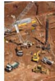
Johannesburg, Gauteng province: Construction in progress on Park Station, set to be the main terminal of the Gautrain rapid rail link. Photo: Chris Kirchoff, MediaClubSouthAfrica.com.
